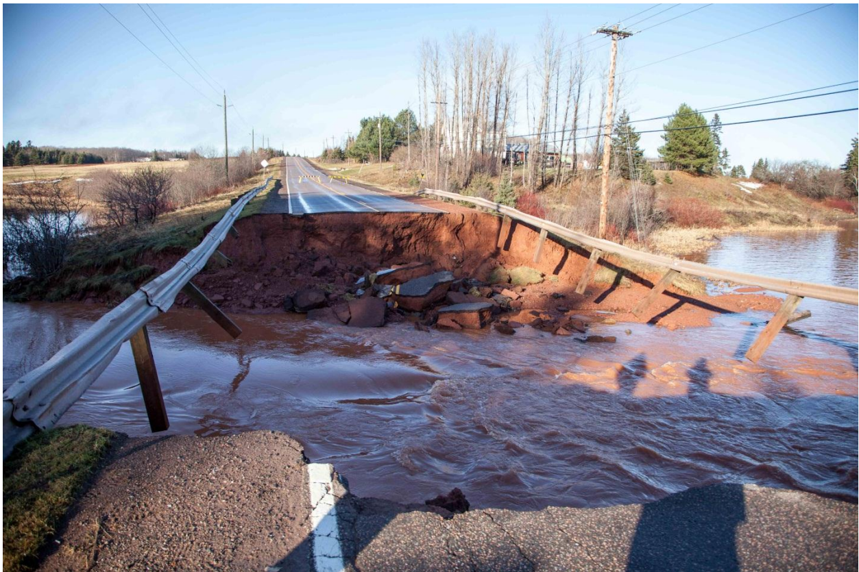
Figure 1 Road Washout at Huntley, PEI – December 10, 2014
