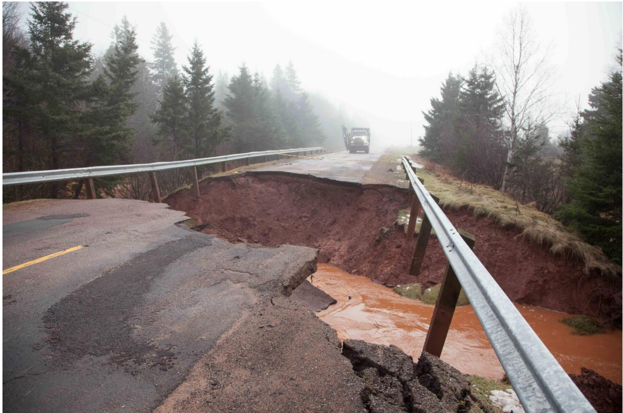
Figure 1 –Lecky Road Washout, Milburn, December 2014
